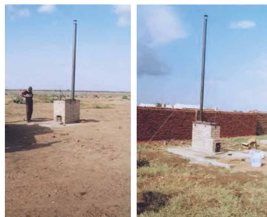
Figure 15 - Photos of double-chamber incinerator
