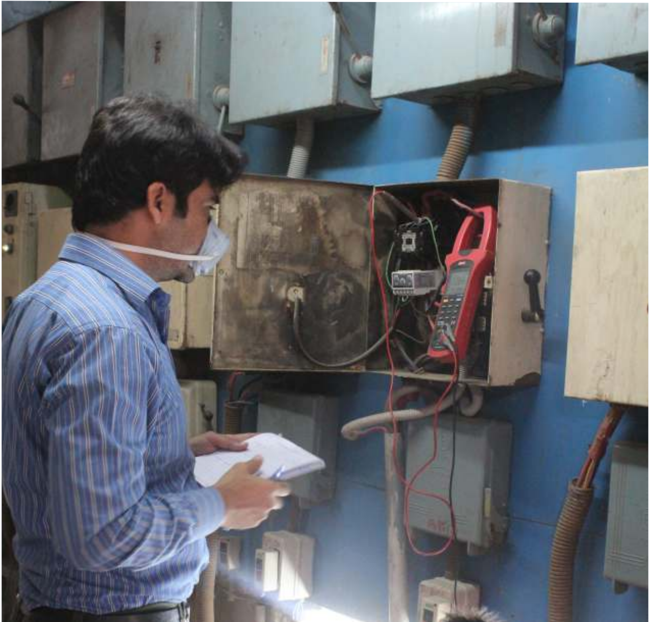
Monitoring of electricity consumption
