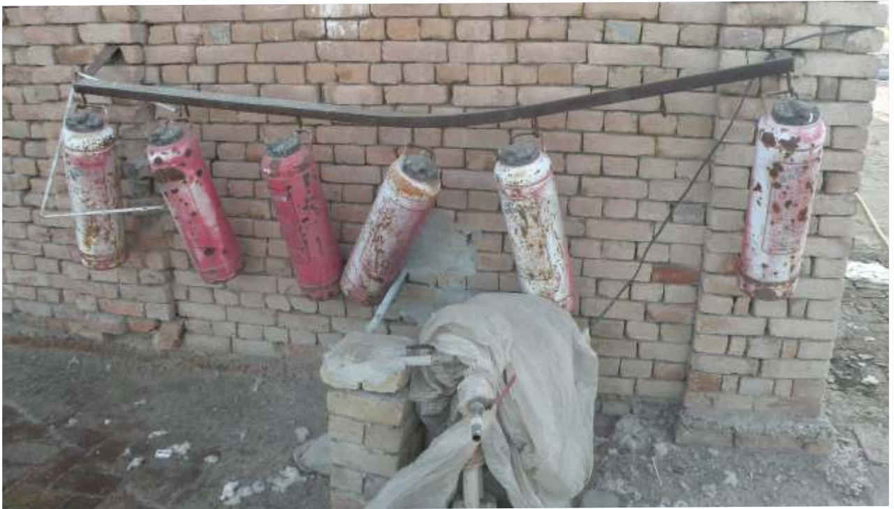
Fire Extinguishers in Poor Condition
