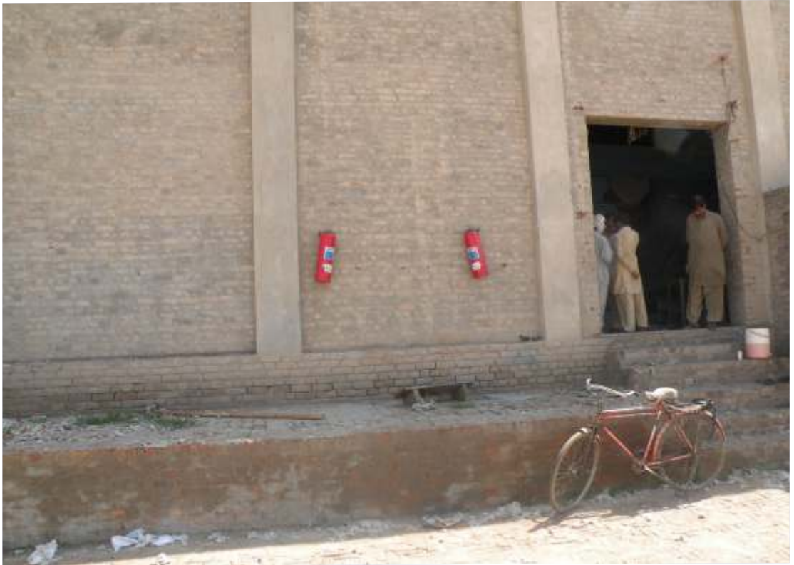
Fire Extinguishers Placed outside ginning Hall
