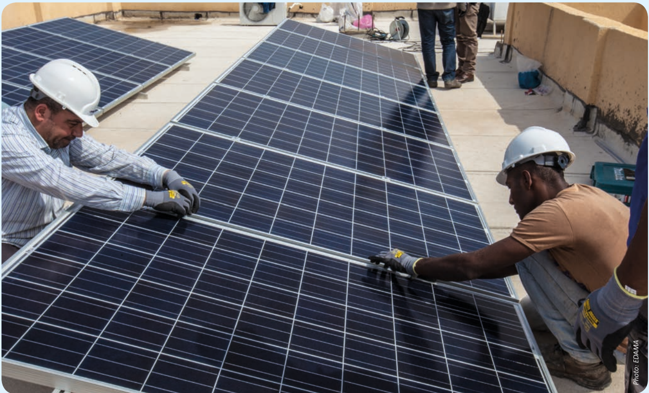
Staff of EDAMA, a Switcher that promotes the effective management of water and renewable energies in Jordan, install photovoltaic systems in a poor village.
