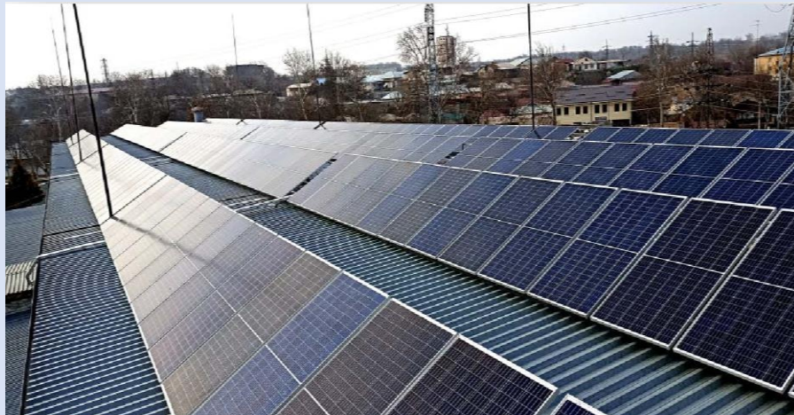
Figure 14. JSC "MAXAM - CHIRCHIQ", Chirchik, solar power plant capacity 100 kW
