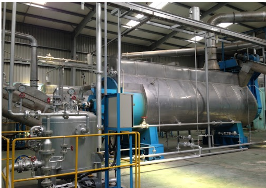
Fig. 10. The thermal oil boiler system
